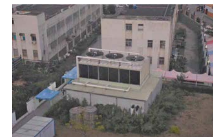
Water cool storage air-conditioning
