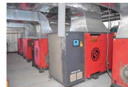
New frequency conversion air compressor
