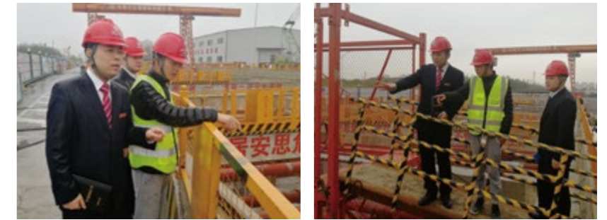
A customer manager of Shaoxing Branch visited the construction site of Shaoxing Metro to see what the customer needed
