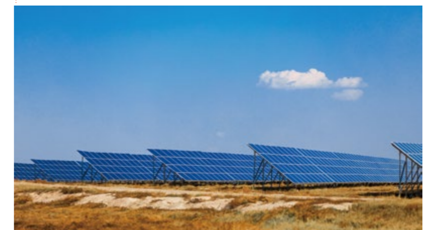
Photovoltaic project supported by the Bank
